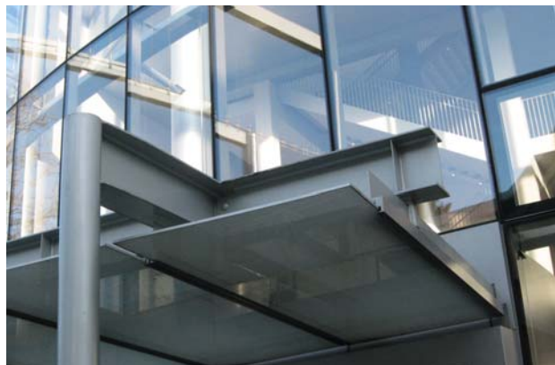
Recent architectural vocabulary tends to use large amounts of glazing and steel. The transparency helps activate the campus and blur the distinctions between outside and inside.
